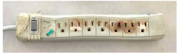
This power bar was placed on the floor in an office in Chernoff. A water spill caused flames to spray upwards into the bottom of a desk.
